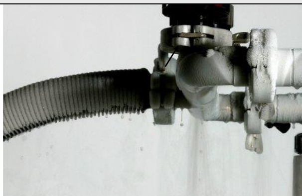
Figure 19 Cold manifold showing drips of liquid air
